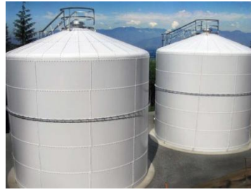
fixed roof tank
