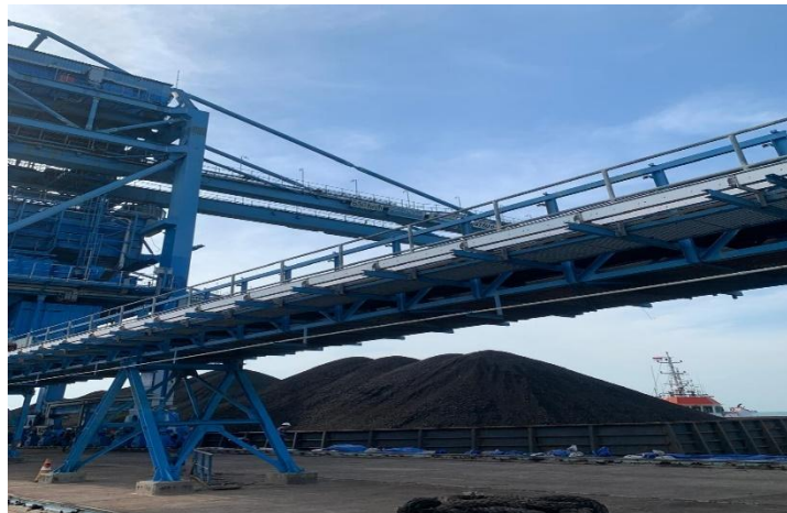
Gambar 3. 1 Conveyor Coal Handling Area
