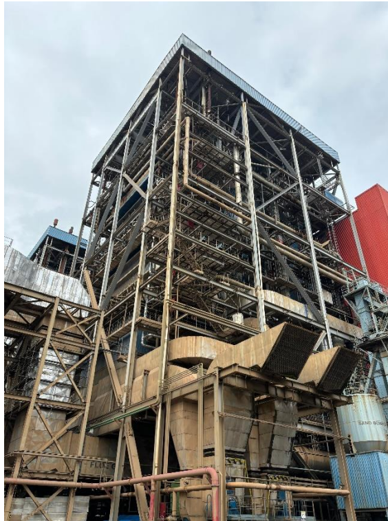
Gambar 3 Boiler CFB PLTU Teluk Sirih[9].
