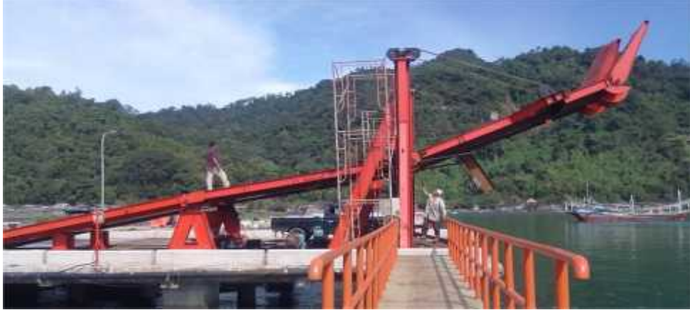
Gambar 4.4 Proses Loading Ramp Gate Door
